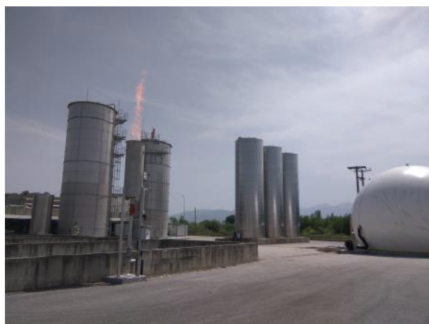
Fig. 1: Picture of an anaerobic wastewater treatment plant in the milk processing industry that SIRMET is designed, constructed and tested for LA FARM S.A. The unit was delivered in April 2017.
